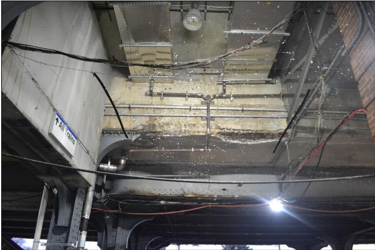
Pigeon netting with feathers and other debris over a pedestrian walkway at Valley Stream station.
