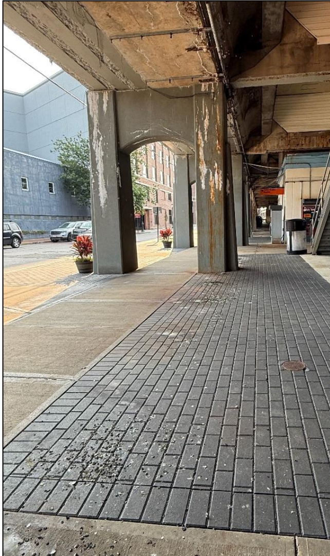
Pigeon droppings at Lynbrook LIRR station.
